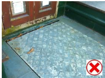
Gaps in the intended slip-resistant paint coatings caused by wear are greater than 75mm and as such this deck area is not compliant.
