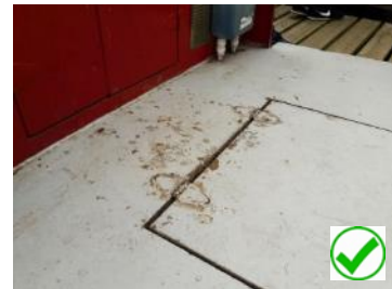
Although the slip-resistant paint coating has worn the areas of wear are less than 75mm across and as such this deck area is compliant.
