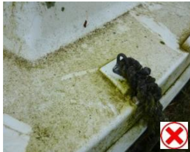
Algae/organic contamination on a GRP moulded deck surface.
