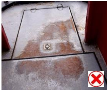
Gaps in the intended slip-resistant paint coatings caused by wear are greater than 75mm and as such this deck area is not compliant.
