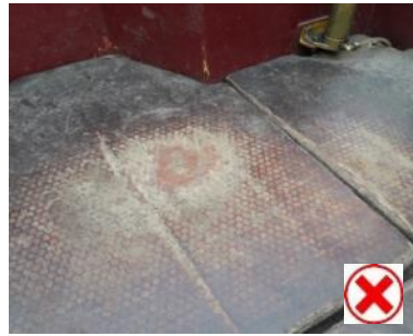
Gap in the intended Hexa Grip board slip-resistant surface caused by wear is greater than 75mm and as such this deck area is not compliant.
