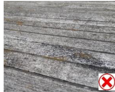
Algae/organic contamination on a teak deck.
