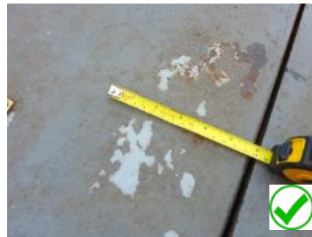
Although the slip-resistant paint coating has worn the areas of wear are less than 75mm across and as such this deck area is compliant.
